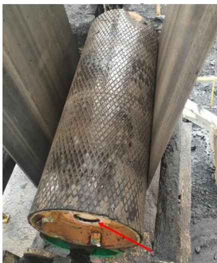
Figure 2 The condition of the HT bend pulley falls over the take-up pulley and counterweight
